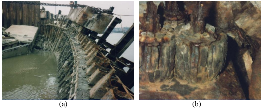
Figure 2: Failure of anchored quay wall (b) corroded barrels and wedges in anchor head (c) lack of corrosion protection behind anchor block [7, 11]
